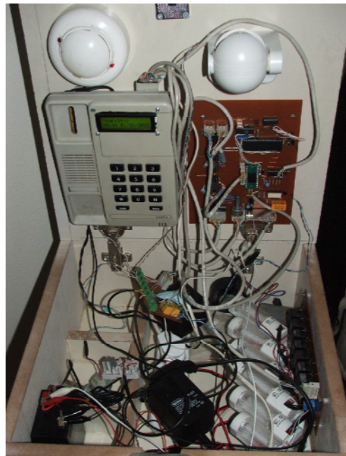
Figure 2. Telephone controlled home automation system
