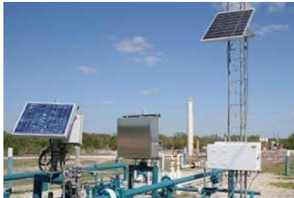
Remote terminal unit
