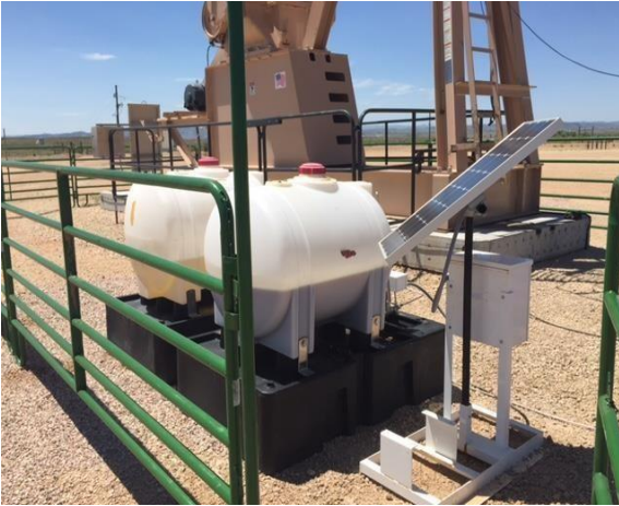
Well monitoring; valves
