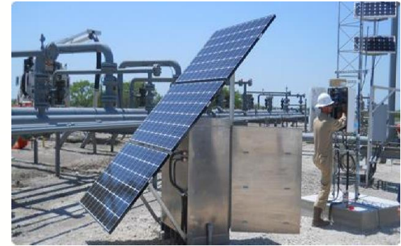
Chemical Injection Pumps
