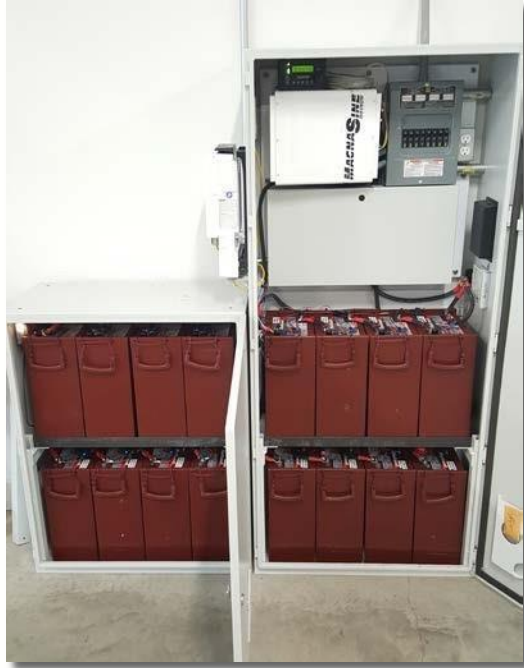
SAGM 06 375 Batteries Minnesota, US
