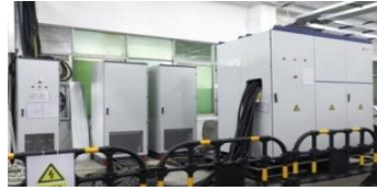
> 6MW Aging Test
