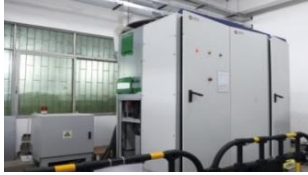
> 3MW Aging Test
