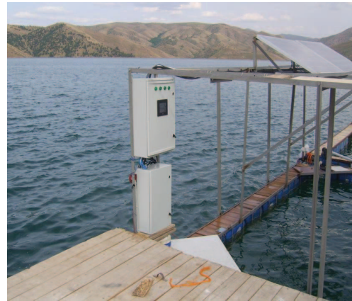
Fig. 9. A view of the designed control panel system
