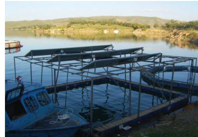
Fig. 3. Developed PV array constructed on the fish cage
